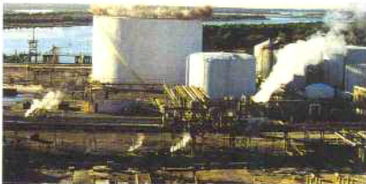
Lake Charles, LA ammonia tank was brought down in a fully operational chemical plant.
