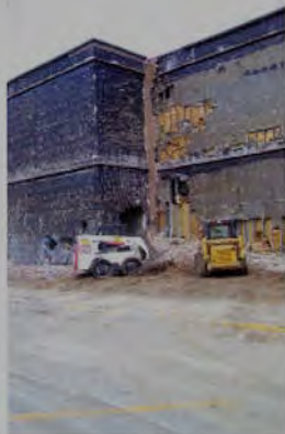
The Graduate School of Biomedical Sciences as brick is being removed at the beginning of the deconstruction process
